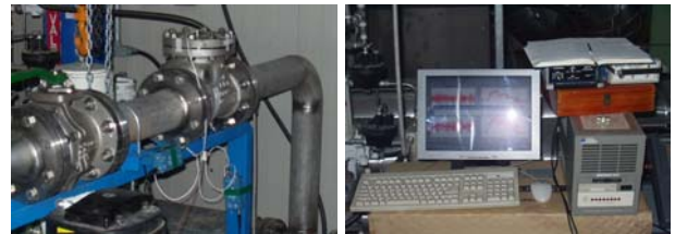
Fig. 6. (a) A 4 inch check valve (b) Experiment instruments
