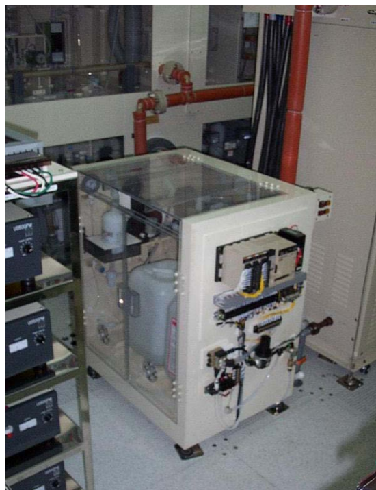
Fig. 5 Developed multi-chemical supply system
