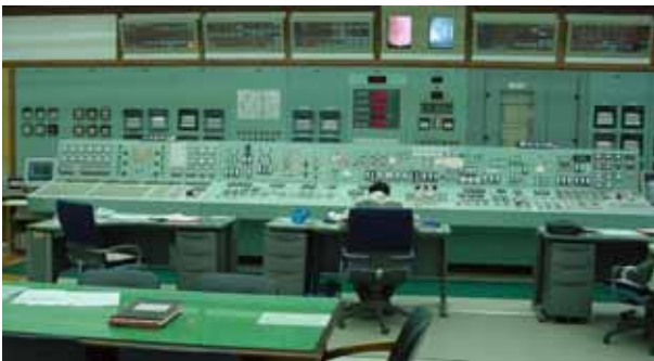
Fig. 8 Image of main control room before retrofitting
