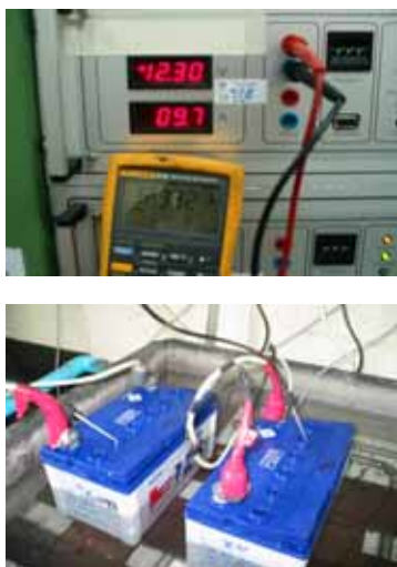
Picture 5 Connecting wire with battery
