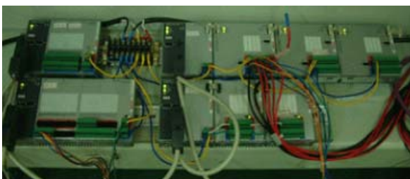
Fig. 2 Distributed I/O modules
