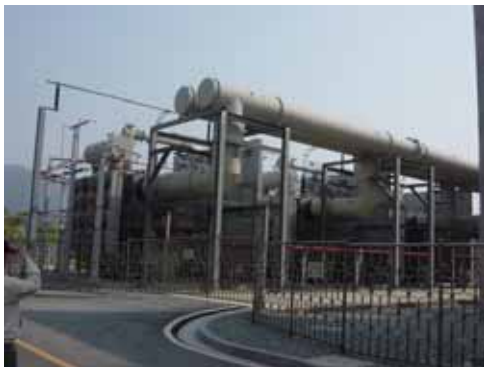
Figure 1. Offsite Transformer (Younggwang 5 unit)
