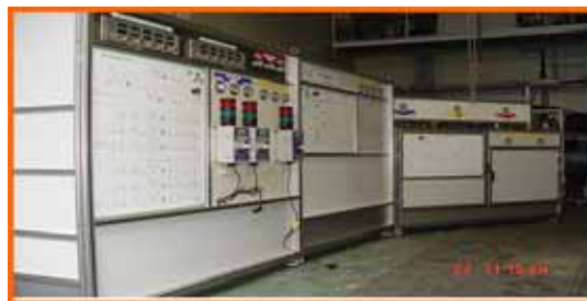
Figure 1. I&C System(GSF-2002) for Fuel Irradiation Tests
