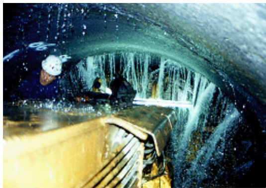
Figure 5. Sketches and Photos Showing Excessive Groundwater Inflow
