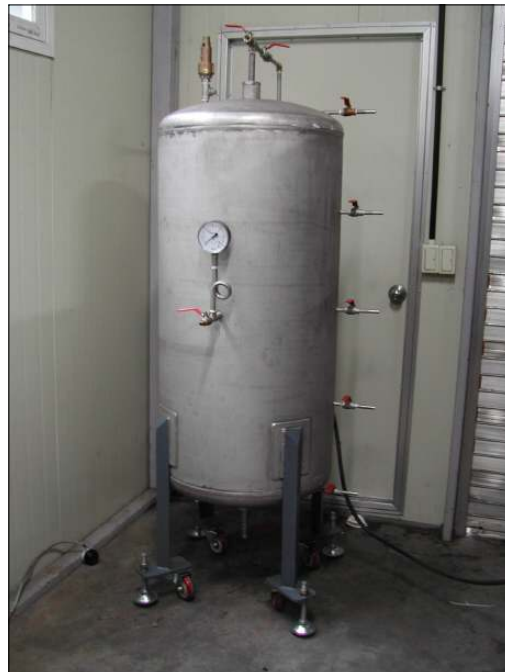
[Figure 1] Storage for gas mixing
