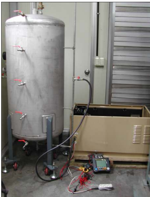
[Figure 3] Gas engine connected to gas tank
