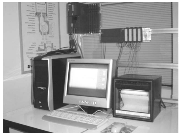
Fig. 5 Control station (PC, PLC and PCI interface card).
