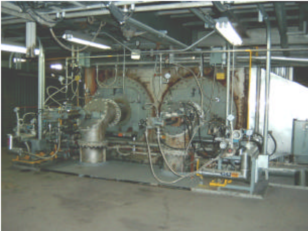
Picture 1 Installed Burner
