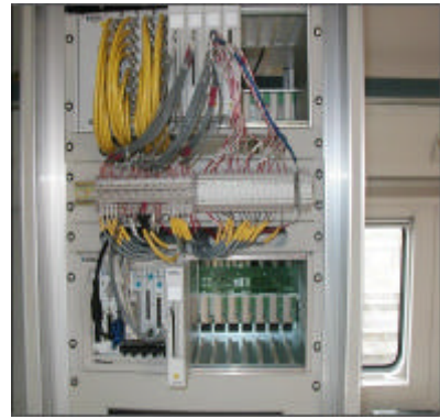
Fig. 4 Data Acquisition system (based NI PXI system)
