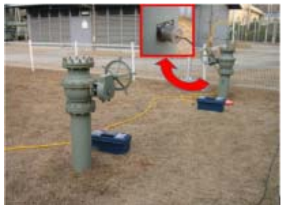
Fig.10 The practical pipeline and the setup accelerometers
