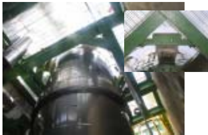
fig. 2 Support type of Secondary Pump
