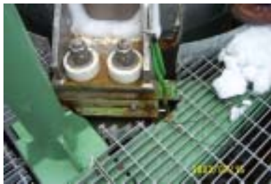
Fig. 4 support point of secondary pump
