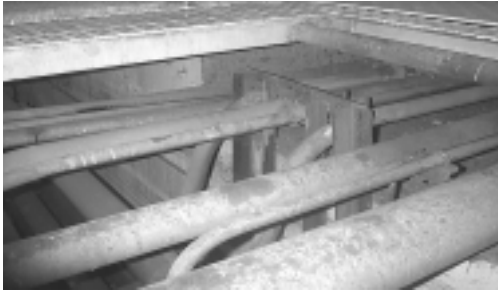
Figure 6. Supported condition of hydraulic oil line
