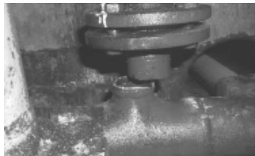
Figure 5. Damage shape(II) of hydraulic oil line
