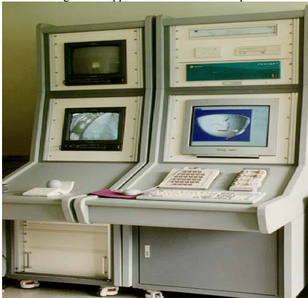
Fig. 9 The supervisory control console of nozzle dam installation/removal robotic system.
