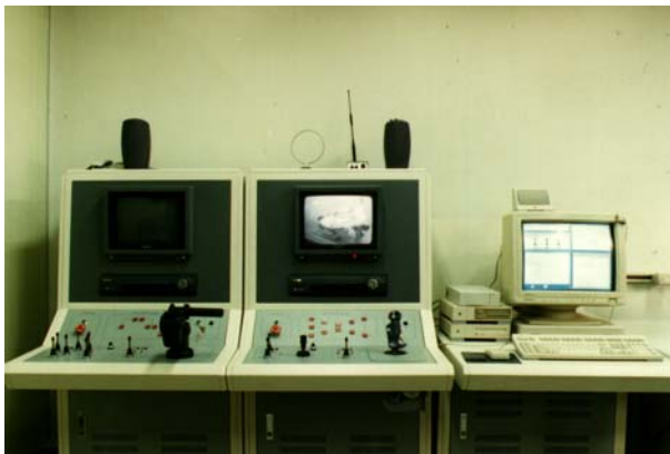
Fig. 12 The supervisory control console of nozzle dam installation/removal robotic system
